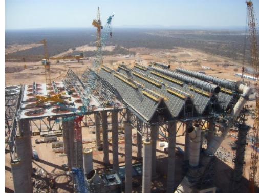
Medupi Power Station Lephalale Customer: Mitsubishi Power
